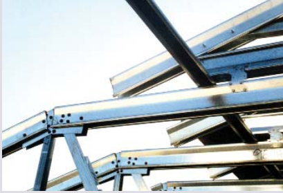
Cap truss installed on top of base truss. Note continuous bracing on top chord of base truss and connection clip.
