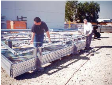
TrusSteel trusses are often light enough for two men to unstack and stage.
